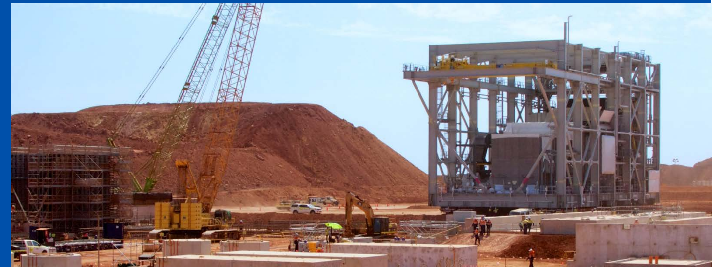
First Gas Turbine Generator
